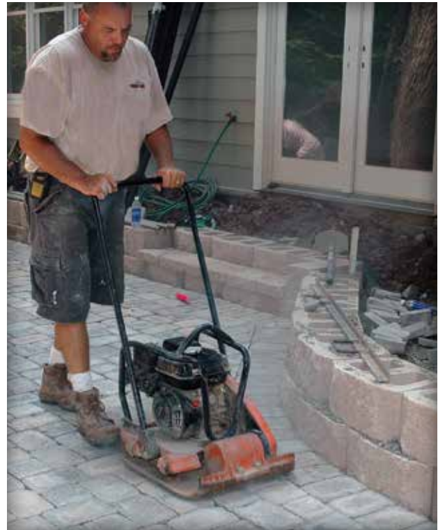
Figure 9. Final compaction of the pavers and settling of the sand into the joints.
