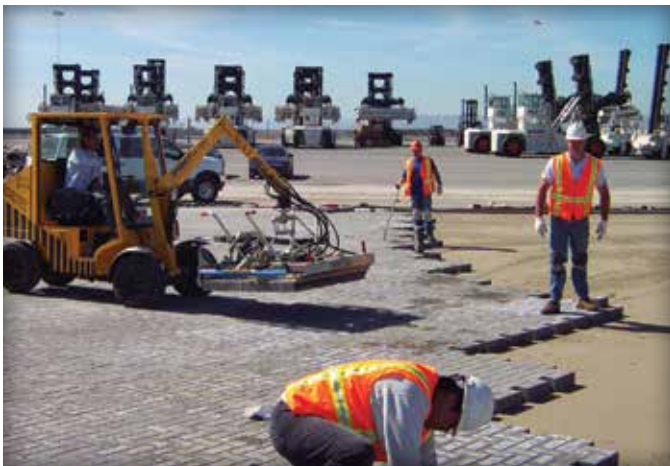
Figure 1. Mechanical installation equipment at Port of Tampa, Florida.
