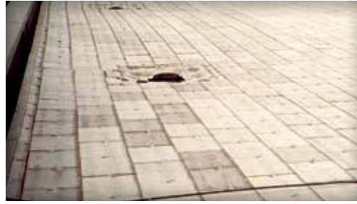
Figure 4. Some ballast-type slabs for roof decks are made with lightweight concrete materials. They can be joined with tongue-and-grooves and/or with connectors to resist wind uplift. This is one of several designs available.
